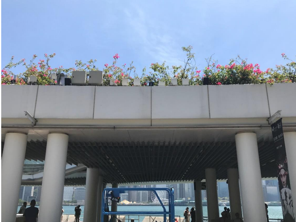
Sample photo of LAA equipment installed at outdoor locations
