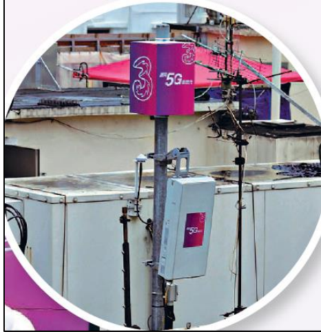
5G AAU on 3.5 GHz band at trial location in Causeway Bay
