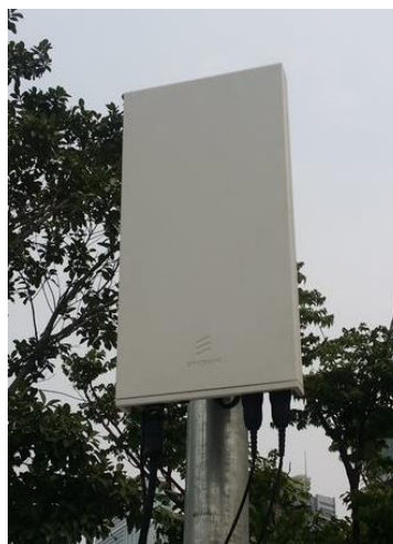
Figure 4. 28GHz Active Antenna on site
