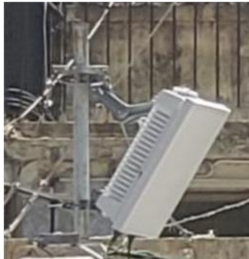
Figure 3. 4.9GHz Active Antenna on site
